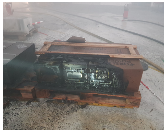
Batteries adjacentes de 7 kWh
